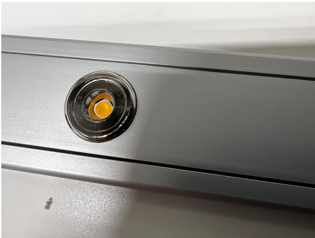
Photo 17 Visual inspection, IPX6. No ingress of water observed behind any of the LEDs.
