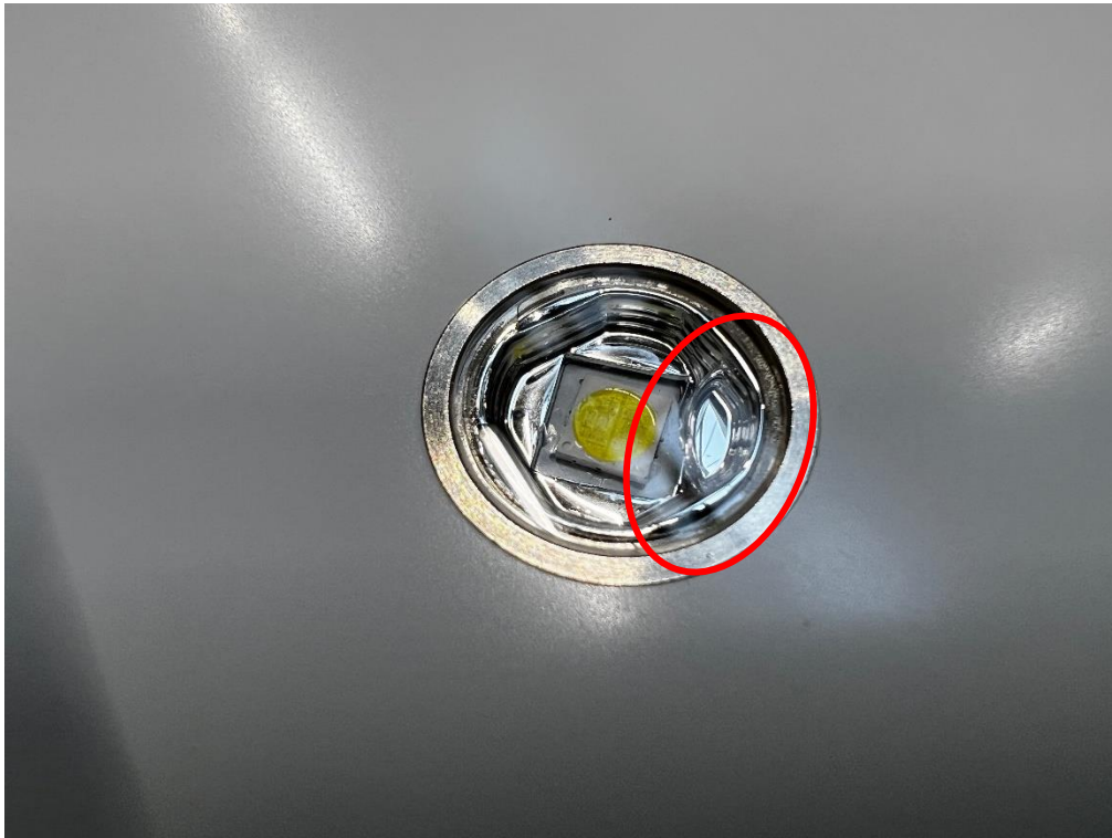
Photo 34 Visual inspection, IPX7. Ingres of water observed inside LED socket (numbered 2 on overview photo).
