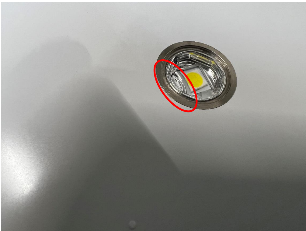
Photo 35 Visual inspection, IPX7. Ingres of water observed inside LED socket (numbered 3 on overview photo).
