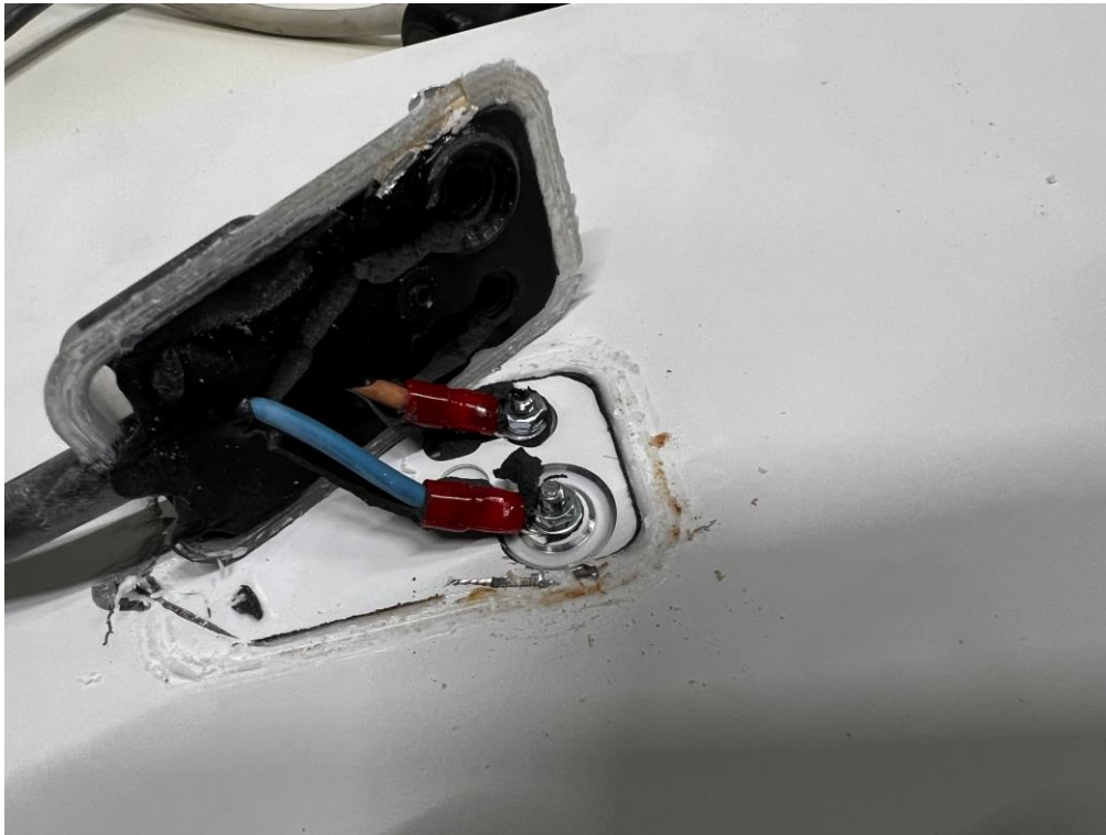
Photo 13 Visual inspection. IP6X. No dust observed inside power connection.
